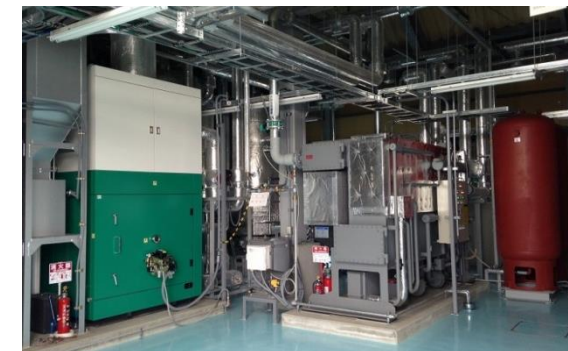
Wood chip boiler
