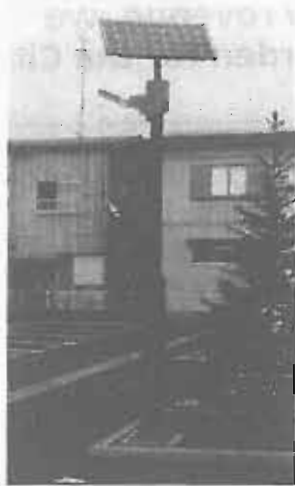
Lighting with a solar panel
